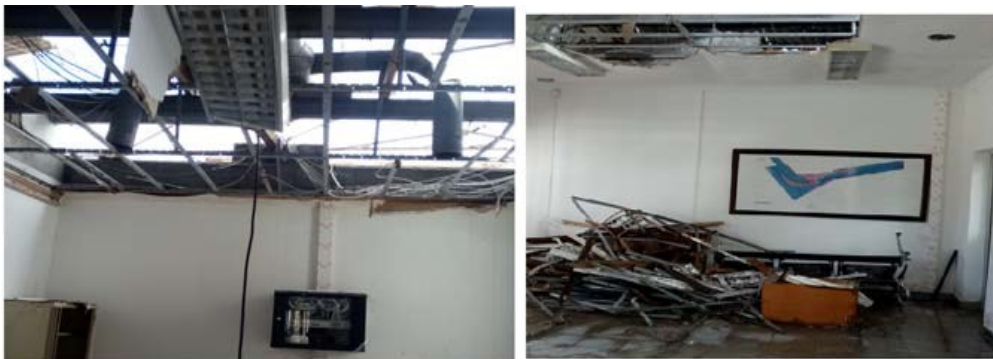
Figures 6: Illustration of the INAHINA's Office upon the occurrence of cyclone Idai. From the figure it is possible to see the damages on the computer equipment, ceil, and furniture.
