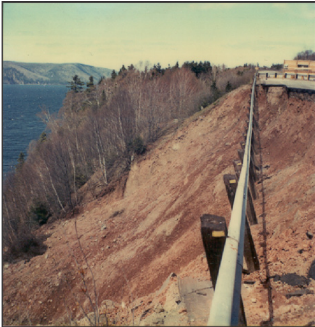
Figure 9. Debris-flow deposit at Kelly's Mountain, Cape Breton Island, Nova Scotia. This landslide has been characterized as a translational failure that developed into a debris flow.
