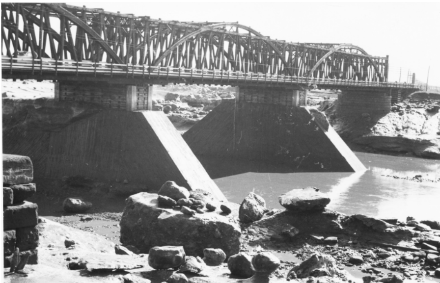
Fig. 54 Same location as Fig. 51, 8 April, 1959. The thaw set in on 30 March, enabling the tide to reach locations at higher elevations. Most of the ice coating is gone; some "toadstool" formations remain, showing that some ice remains bonded to the banks. Banks and ice are covered with a layer of silt. Photograph #459-3.
