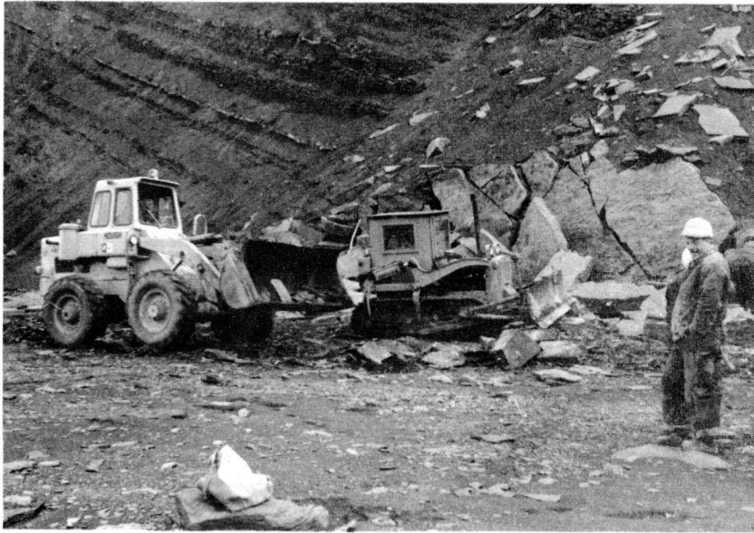
Figure 1. A bulldozer and payloader prepare to remove the track-bearing slabs (on right) from the bottom of the Joggins cliff.
