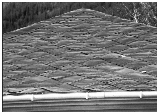
Fig 8 Example of fuel cans reused to shingle a roof in Dawson City. Photo by M. Gates.
