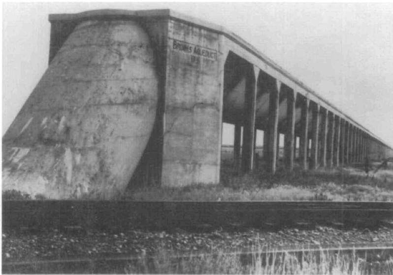
Fig. 1 Siphon outlet of the Brooks Aqueduct, ca 1950, one of the images appearing in the exhibit. (Courtesy Provincial Archives of Alberta)
