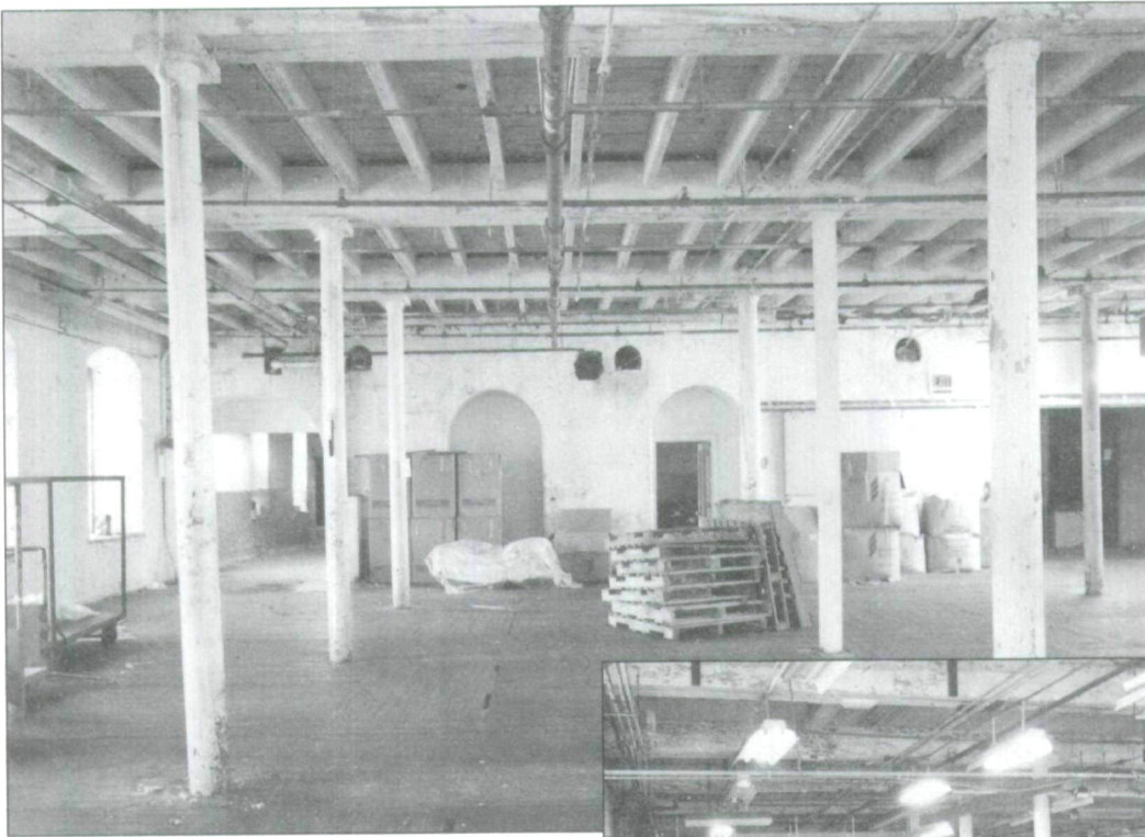
◀ Fig. 5 Interior of the third storey of the main block of the Rosamond mill. The joists are a sign that this part of the mill predates the introduction of slow-burning mill construction techniques. The semicircular holes in the stone wall show where line shafting ran. (Courtesy: Canadian Parks Service, Canadian Heritage Recording Services)
