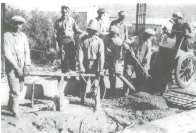
Fig. 2. As a relief project the bridge employed many men from the district as a manual labour force. This 19 September 1936 photo shows workers pouring concrete for the road slab. Note that two vibrators are being used to assist in spreading the concrete. (Photo: Private collection.)
