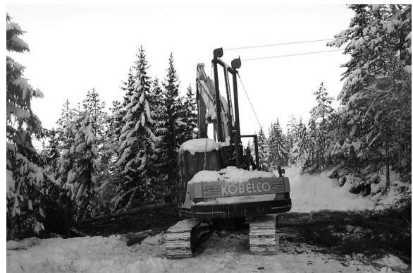
Figure 5. The prototype excavator with tower and processor is able to rotate under the skyline when processing and sorting timber. The machine can move in any direction to organise logs along the roadside or to position the skyline.
