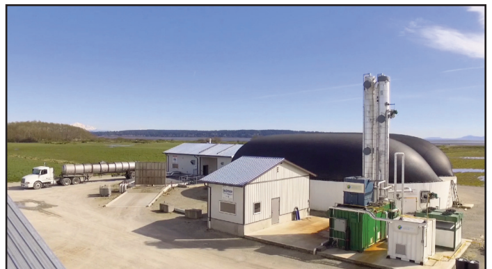
Seabreeze Farm Renewable Natural Gas plant, Delta, British Columbia (Photo: Greenlane Biogas).
