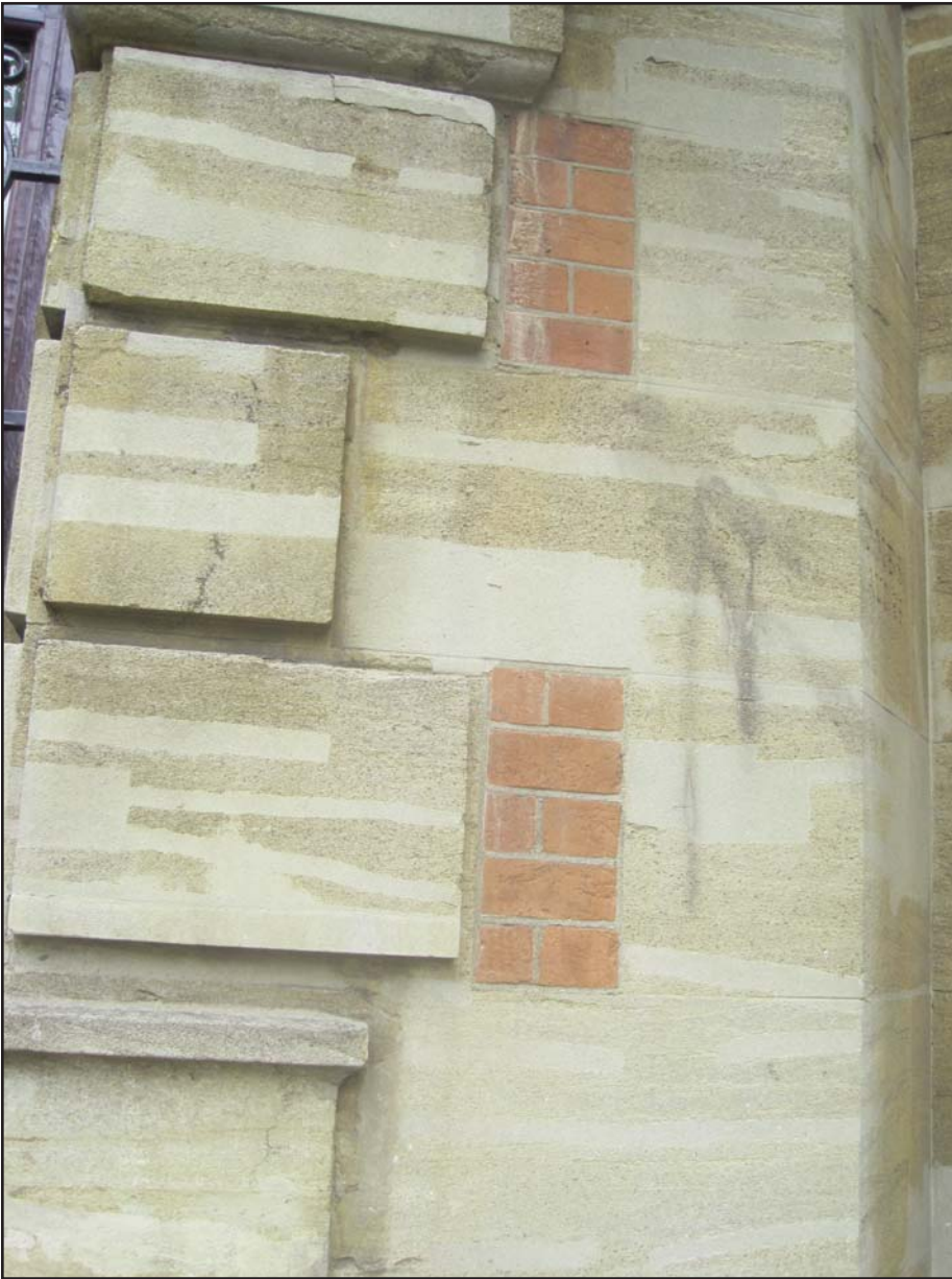
Figure 7. Part of the façade of a bank in Hampstead, London, showing inappropriate use of cement and brick in repairs to Douling Stone.
