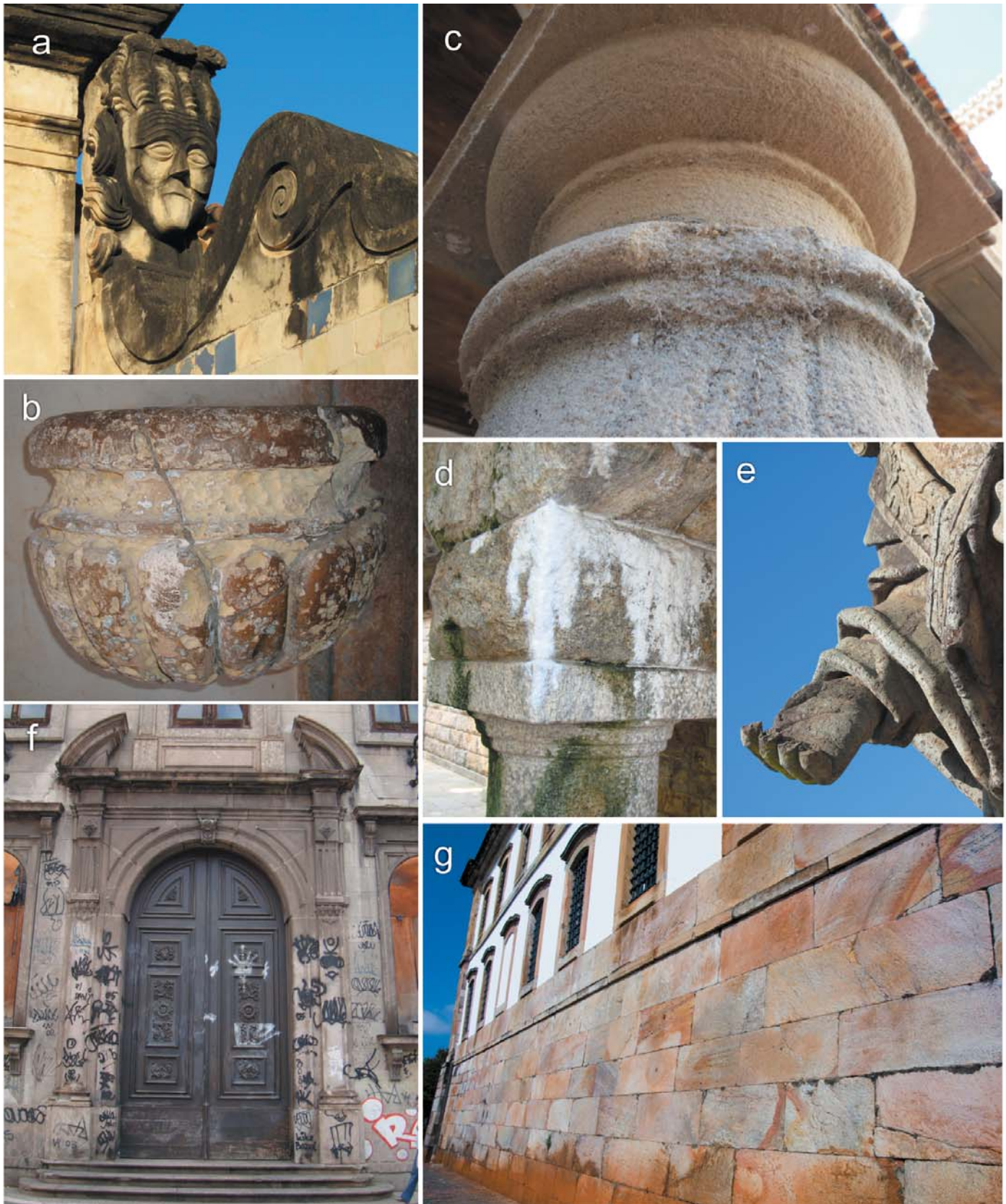
Figure 3. Examples of damage that attest to some of the processes responsible for decay or alteration of the stone in some historic monuments built in Brazil. a) Biological colonization and black crust on limestone in the São Francisco's Convent in João Pessoa (state of Paraíba); b) crack and alveolization of limestone in the Church of São Pedro dos Clérigos in Recife (Pernambuco); c) disintegration of calcarenite in São Francisco's Convent in João Pessoa (state of Paraíba); d) encrustation associated with gneiss in the Palacete Laje in Rio de Janeiro (state of Rio de Janeiro); e) missing part on one of the prophet statues at the Bom Jesus Sanctuary of Congonhas (state of Minas Gerais); f) graffiti on the Church of Santíssimo Sacramento in Rio de Janeiro (state of Rio de Janeiro); g) patina formed on quartzite in the old Chamber and Prison House in Ouro Preto (state of Minas Gerais).
