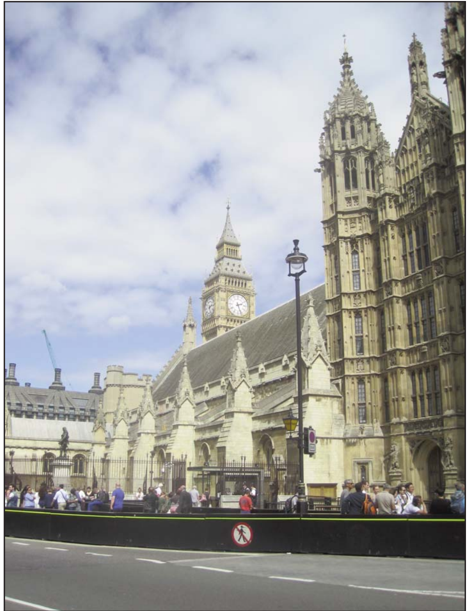
Figure 2. The Palace of Westminster showing pale-coloured Clipsham Stone from recent repairs, contrasting with Clipsham Stone from previous repairs and Anston Stone.
