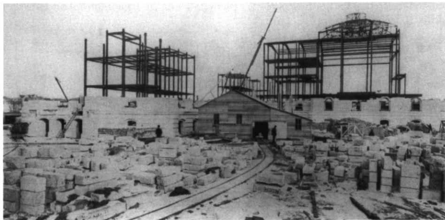
Figure 4 Storage area on the southwest side of the Legislature for sandstone blocks and bricks. The narrow gauge railway ran from the spur in Figure 6 into the cutting sheds visible in the middle distance. The elaborate steel skeleton of the Legislative Chamber on the south side of the building has been erected (Provincial Archives of Alberta, A 11027).
