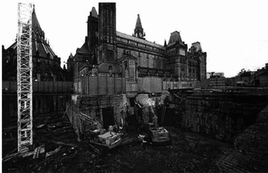
Figure 17 Excavation for the Centre Block Underground Services space (CBUS) involved the removal of about 30,000 m 3 of rock during a 3-month period in 1997. PWGSC 1997.
