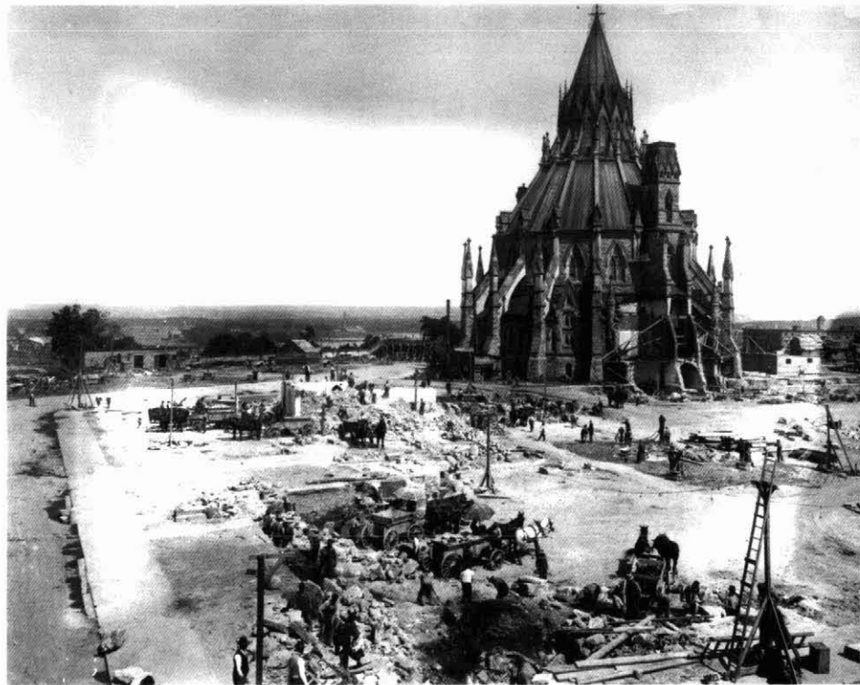
Figure 3 Preparation of Parliament Hill for reconstruction of the Centre Block, 15 August 1916. Workmen with horse teams are removing the last of the rubble from the foundations of the former building. In the middle ground, in front of the Library, another crew is drilling blast holes for foundation excavations. Only the Parliamentary Library remains intact. Its shored up entrance, which connected it to the Centre Block, can be seen beyond the drilling crew. National Archives of Canada PA130624.
