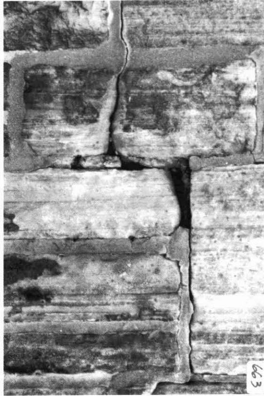
Figure 15 Deterioration of mortar due to freeze/thaw cycling. Note the adjacent Nepean Sandstone, heavily soiled in part, has also suffered. Cracked mortar and stone facilitated further entry of moisture. PWGSC, 1995.
