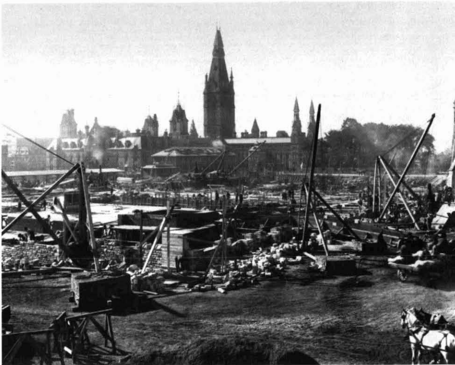
Figure 4 View looking southwest showing the early stages of the reconstruction of the Centre Block. Beyond the construction on the left is the stone cutting shed and to the right the architect's offices. The West Block is in the background. Photo taken 26 September 1916. National Archives of Canada C6361.
