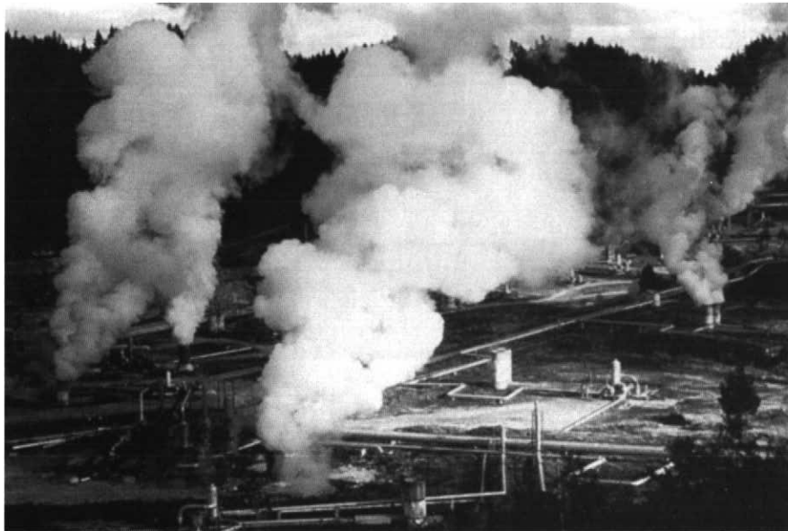
Figure 3 The well field at Wairakei, New Zealand, where wells have been drilled into a hot-water reservoir. The two-phase mixture is separated into its components in the separators, the small cylindrical objects. The large cylinders are noise mufflers for waste discharge.
