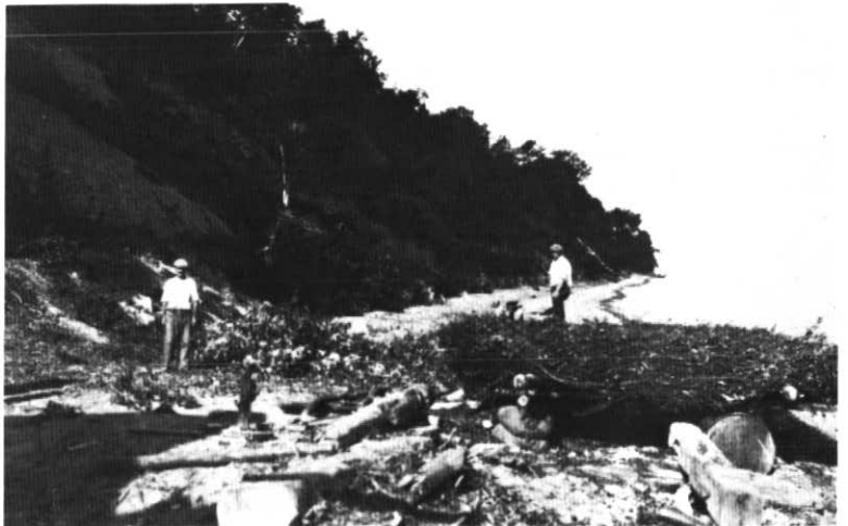
Figure 7 Early attempts at remedial work: "Mississippi mats" constructed by laying brushwood, mostly willow, on a wooden frame, being placed around the intake for the Scarborough Waterworks (Fig. 3) in the mid 1930's (from the collection of A.P. Coleman)
