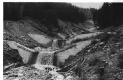
Figure 7 New check-dams along a deeply scoured source area of residual colluvium near Inzing, Austria. These dams, arranged in a stacked pattern, confine the torrent to a central line and create a more balanced profile, thus preventing erosional instabilities along the embankments. Note the gently rising stone carapaces on either side of the discharge section of the check-dams; they are designed to accommodate the passage of small debris flows without endangering the lateral abutments.
