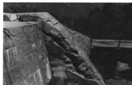
Figure 8 Wing of a check-dam, being slowly crushed by lateral pressure resulting from deepseated creep along unstable flanks of a torrent channel near Crodo, Italy.
