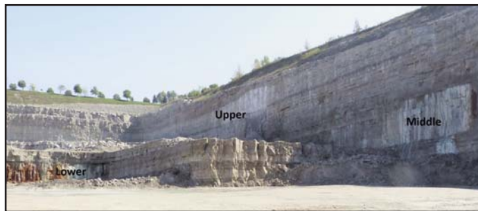
Figure 17. Inflow of sulphur water along bedding plane partings in the Lucas Formation on the southern face of the McGregor Quarry. Inactive zones are marked by white residue immediately below the bedding plane. The red staining on the lower bench marks an active inflow with a rotten egg smell, indicative of the presence of sulphur-oxidizing bacteria. Exposed bedrock thickness is approximately 40 m. Photograph taken October 18, 2013.
