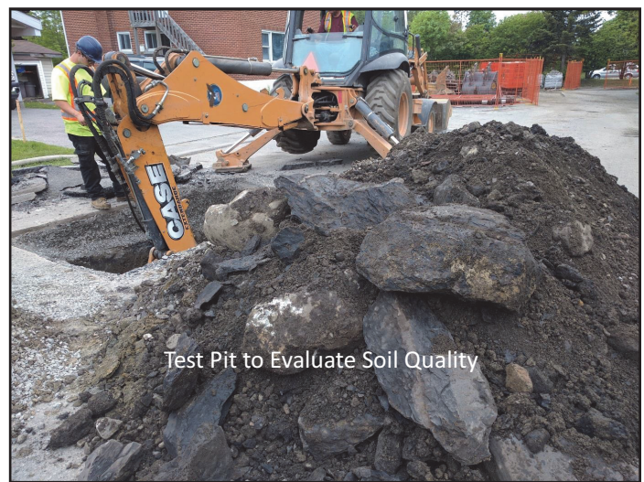
Figure 4. Example of test pit excavation to assess soil quality in the area of infrastructure renewal in Case Study #3.
