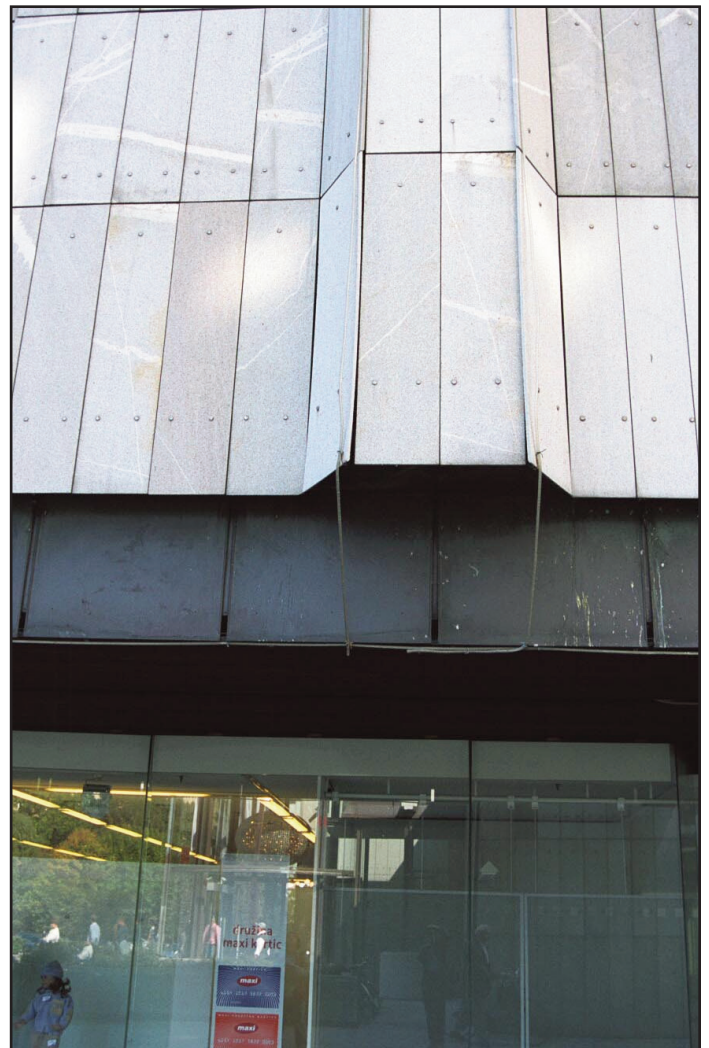
Figure 8. Bowing of granodiorite on a building façade. Photo: Ana Mladenović.
